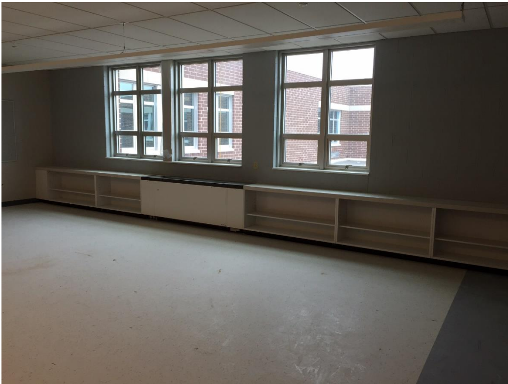
Classroom metal casework
